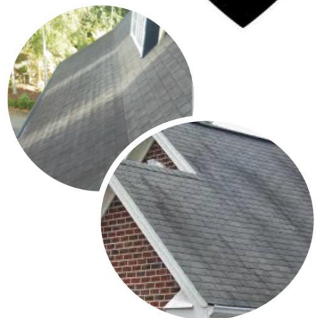
ALGAE STAINED ROOF
